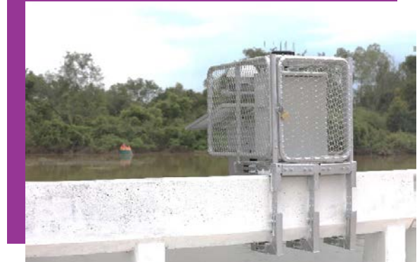
Automated telemetry station on the bridge
